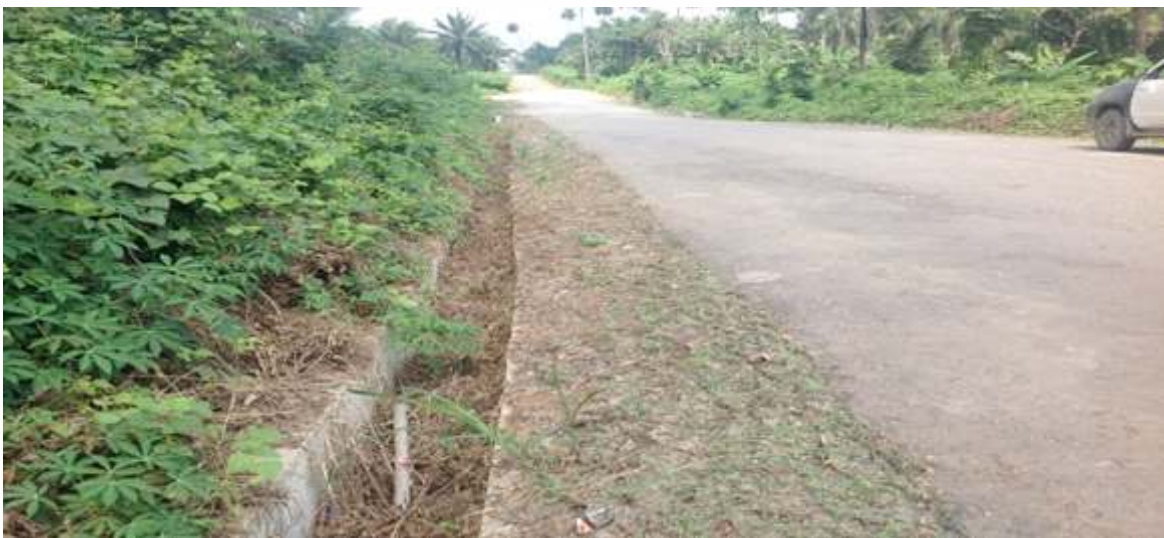
Section of Lot 2 Phase I, with drainage system in Okoyong-Usang –Iso road, Cross River
