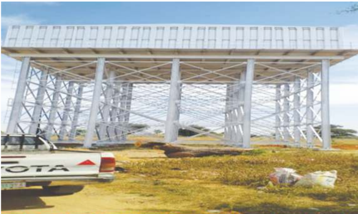
1500 cubic meters Overhead Water Tank at ABU Zaria
