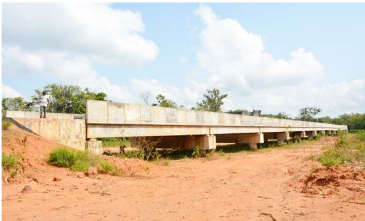
View of the Ovia River Bridge Road Phase 1, Irele LGA, Ondo State
