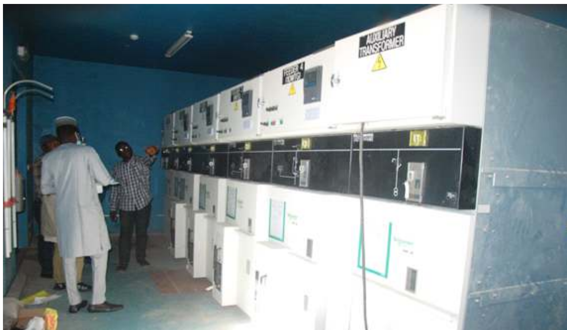
Internal Substation room housing the Switch gears for wind farm Feeders at 10mw Katsina Wind Farm- Katsina State
