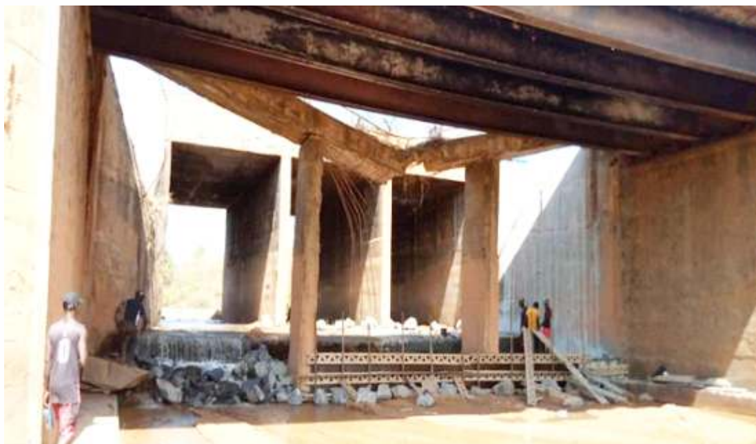
Emergency works at Laftagi Bridge on Ilorin – Jebba – Mokwa/Bokani Junction Road Section II: Jebba – Mokwa, Niger State
