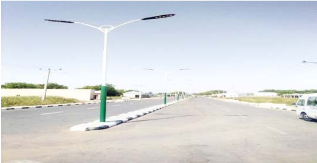
Construction of road networks, walkways and surroundings at FMC Azare, Bauchi State
