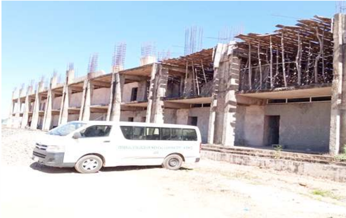
Side view of on-going, two storey research laboratory at the Federal School of Medical Laboratory Technology (Science) Jos
