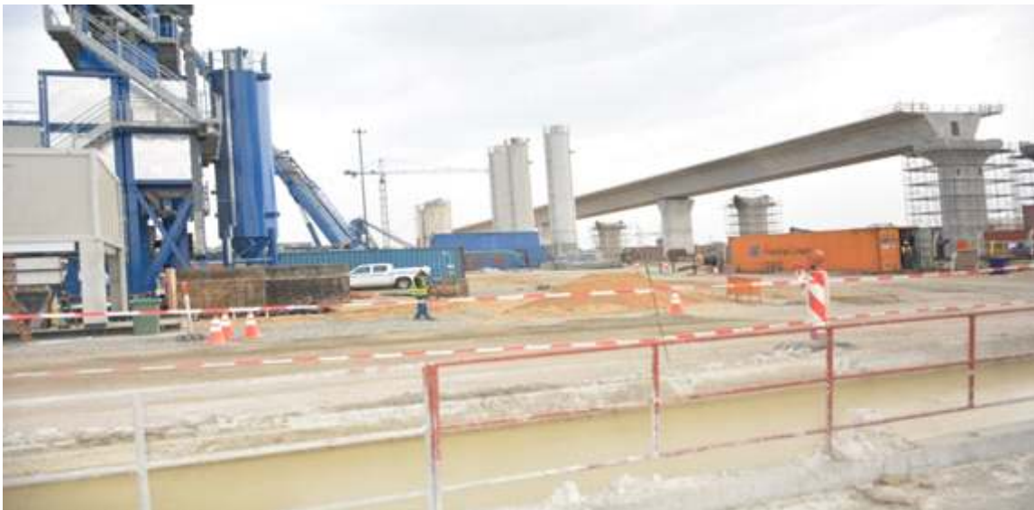
Construction of 2 nd Niger Bridge at Onitsha Linking Anambra and Delta States
